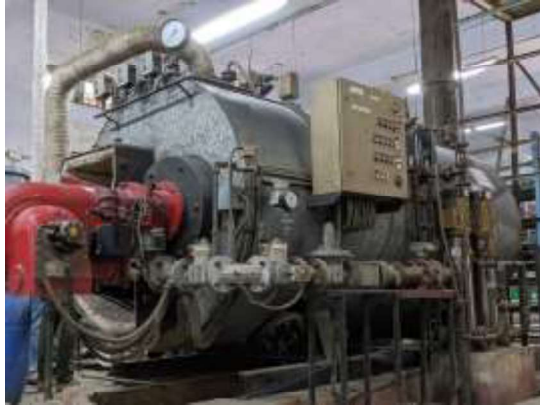
Boiler Laboratory of the Department
